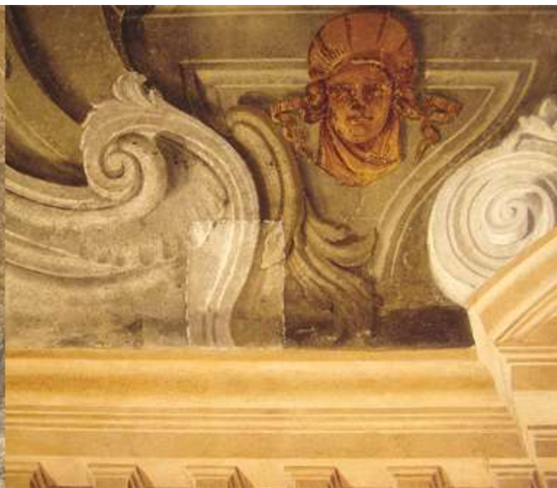
Fig.5 (left) Figure of Council in the Northern wall, before restoration.
